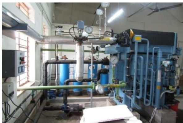
Indoor Refrigeration Unit
