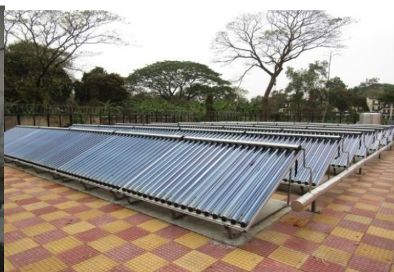
Outdoor Solar Thermal Unit
