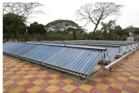
Outdoor Solar Thermal Unit
