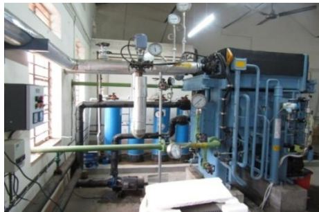
Indoor Refrigeration Unit
